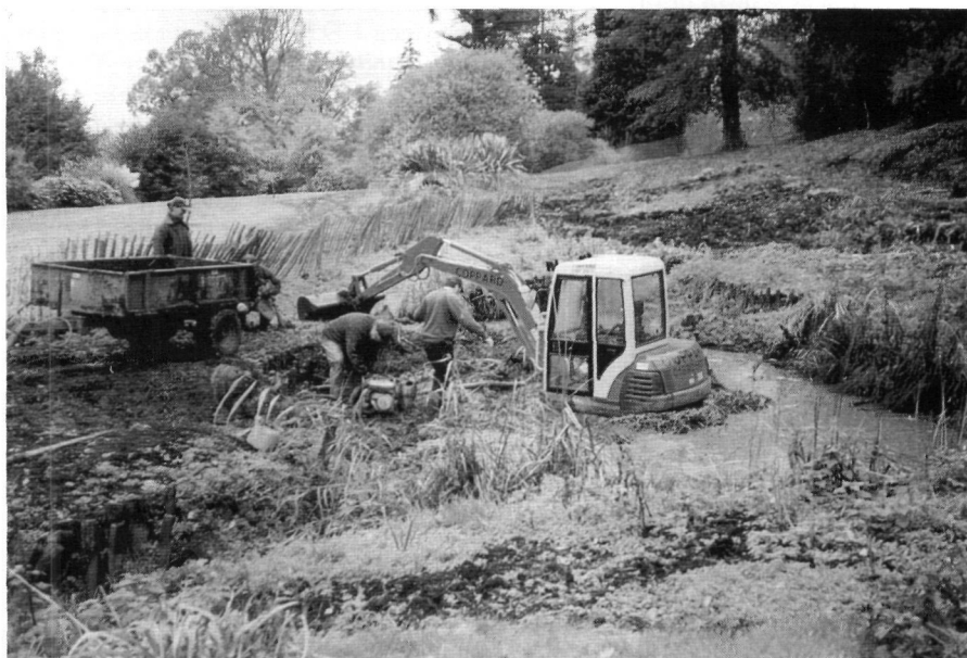
'Man the pumps': progress is slowed by very wet conditions in the Bog Garden. (Photograph by D. Hardman.)
