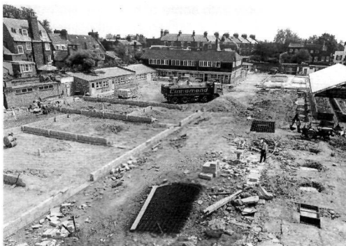
The Melon Yard – the single phase project meant a logistical nightmare. Careful planning overcame difficulties during the demolition and early construction phase.
