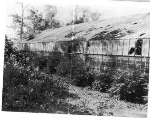
Left: Temporary Palm House damaged by falling poplar branches in October hurricane.
